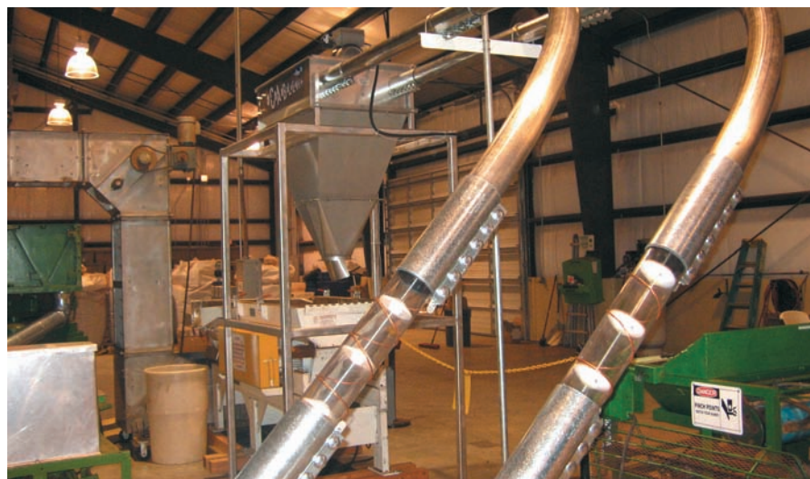
Close-up of Inspection Tube shows tea moving.
