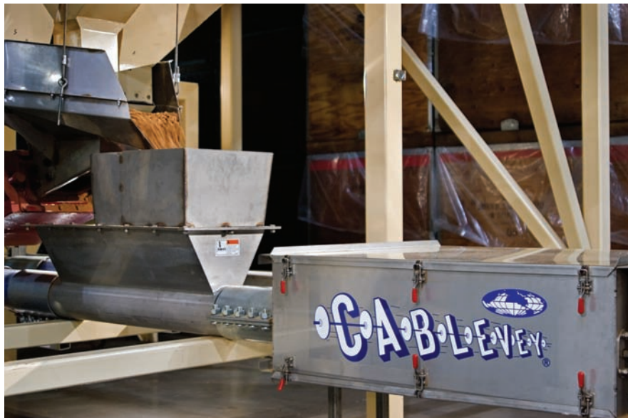
Almonds are discharging from a holding tank into an inlet near the tension turn around unit on one of the tubular drag conveyors.
