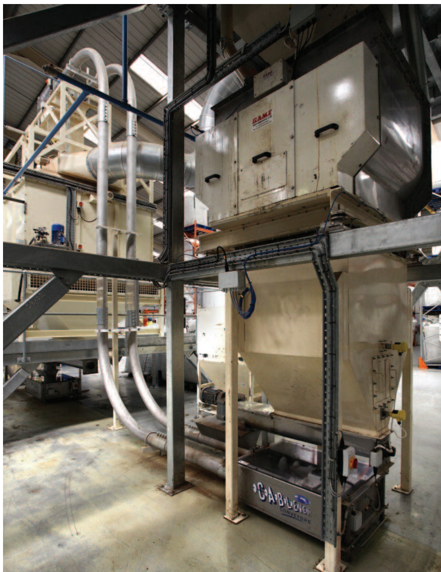
The stainless steel tubular drag cable conveyor provides dust-free conveying from the mixer up to the cooler inlet.
