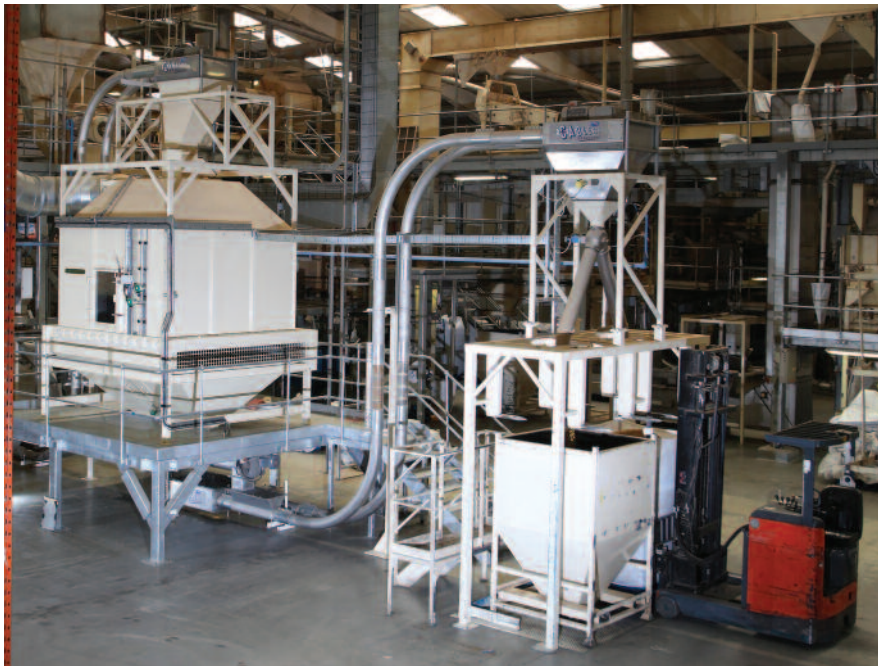
The tubular drag cable conveyor gently moves the pet food from the cooler to the bulk bin at up to 6 tonnes per hour, transferring product without degradation or cross-contamination.
